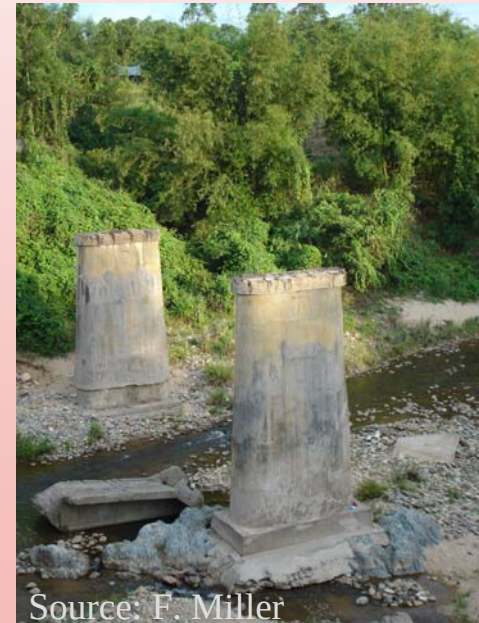
Bridge damaged in 1999 flood
